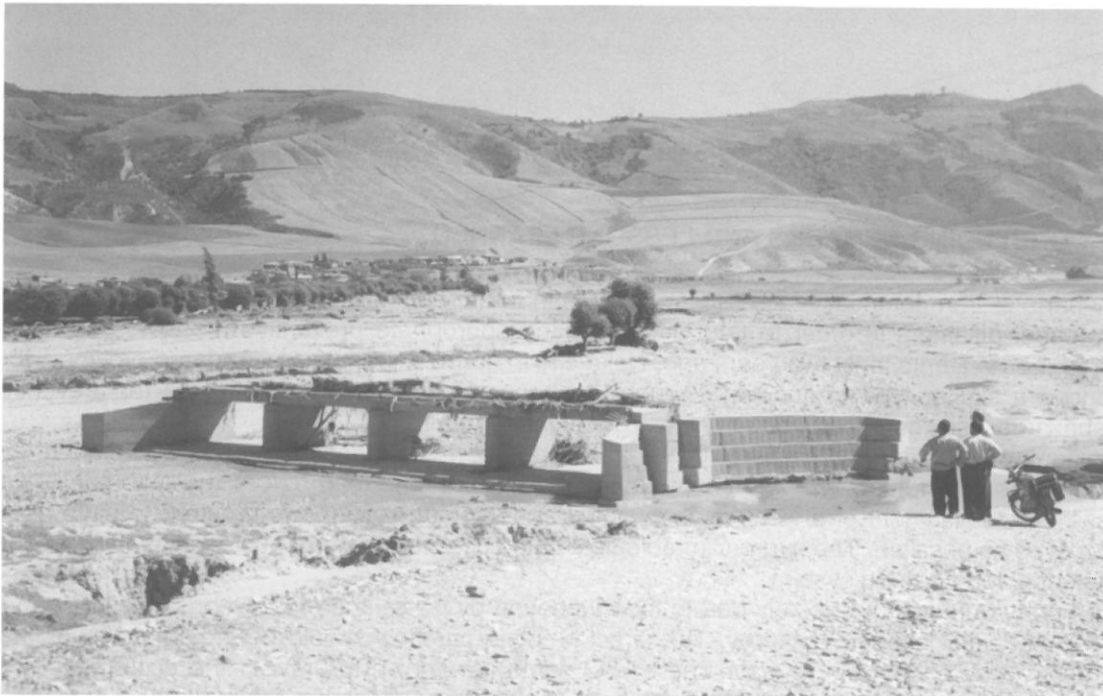
Figure 5-2: Bridge damaged by debris flow.
