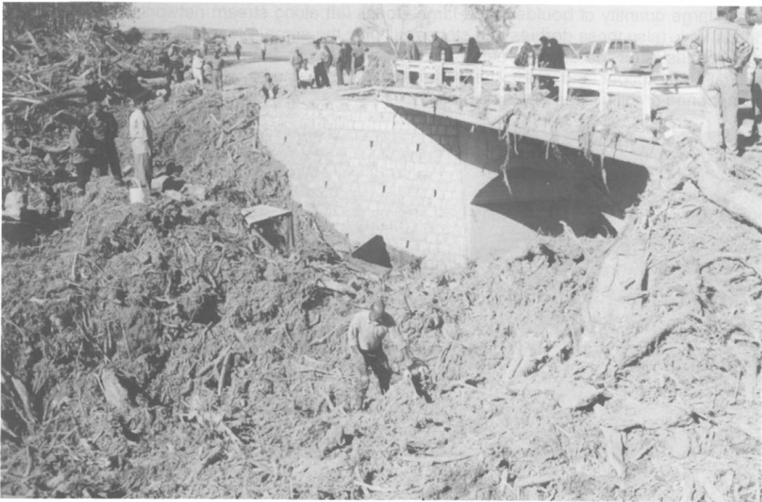
Figure 5-1: Fine sediment carried by flood blocked the water way.
